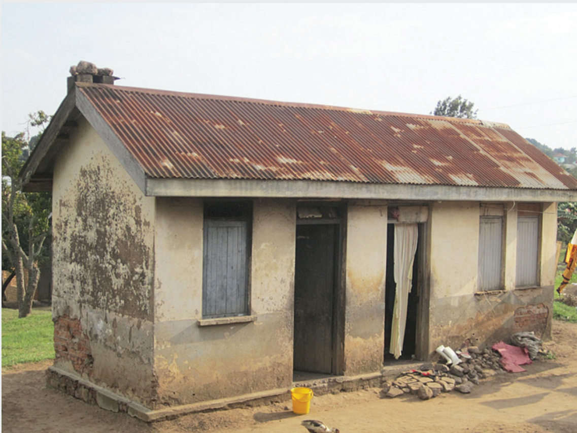
This kitchen was turned into a house for a health worker
