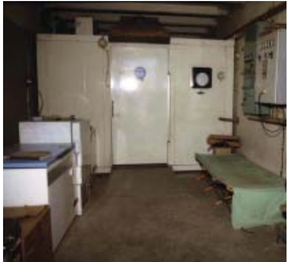
Continuous monitoring of vaccine stocks is needed, as shown in this national cold room.
