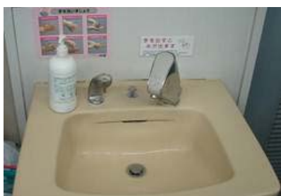
11. Adequate disinfected facilities at the washing basin.
