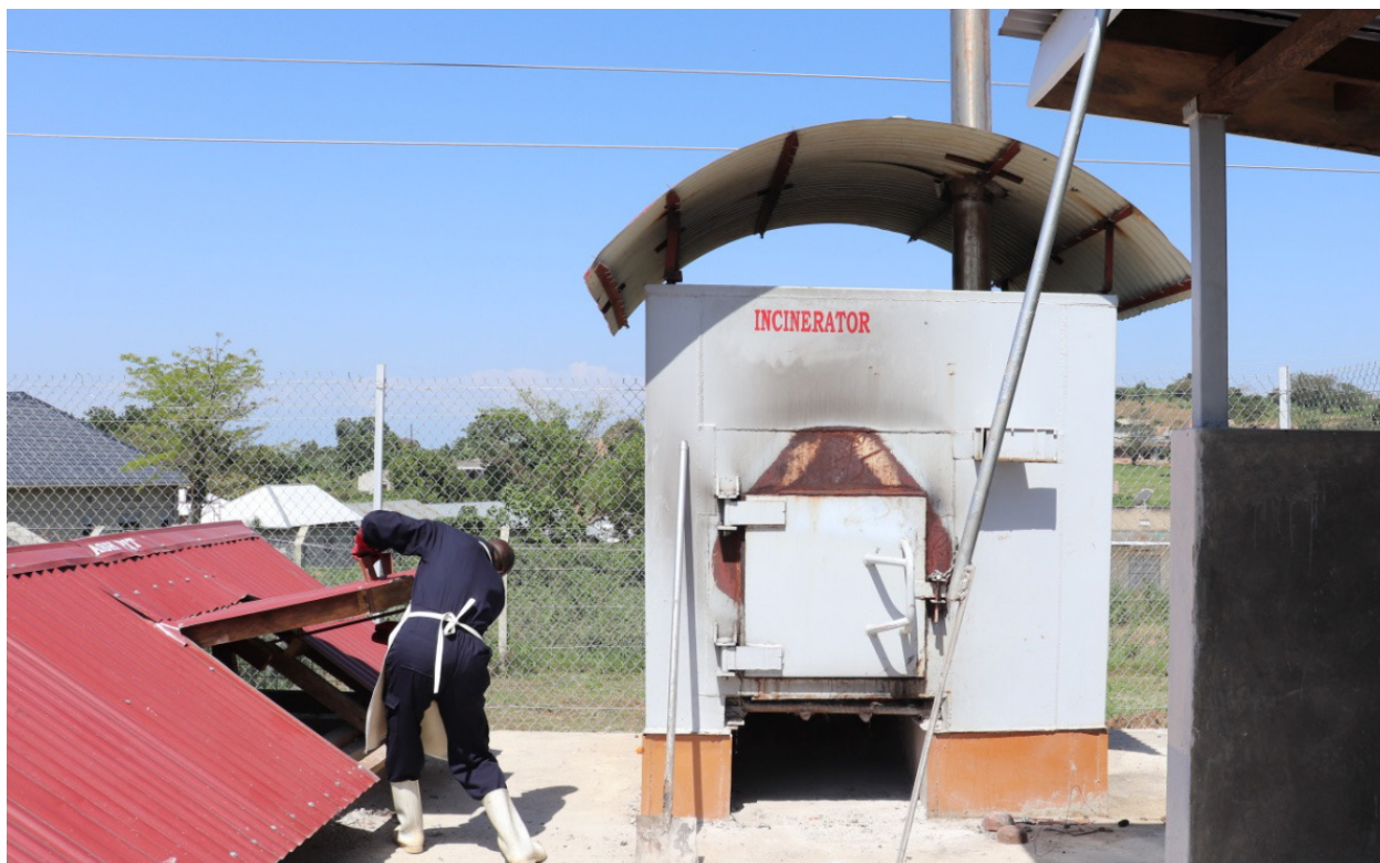
Figure 8.7: Picture of an incinerator and ash pit close-by (Source: Water for People)
