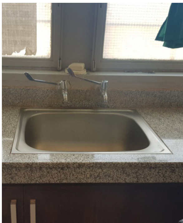
Figure 5.6: Hand washing facility with stainless steel bowl
